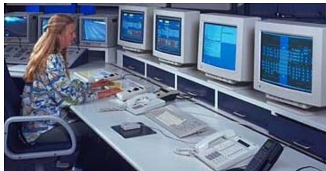
Figure 3.7: Control room of a distributed control system (DCS)
